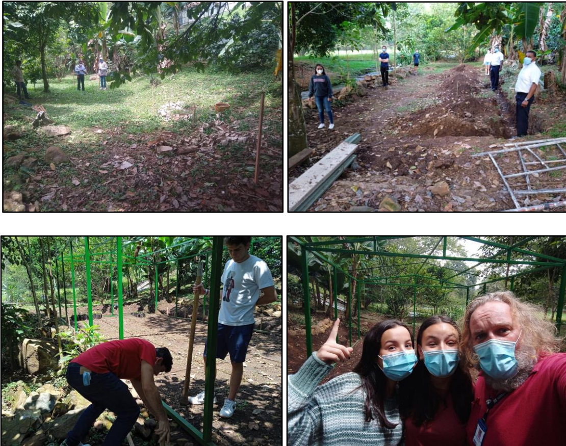
The Bolivar Garden Greenhouse project in process. The original site for the greenhouse was then flattened by the school's gardeners. Funds from a variety of sources including the 5K Verde Race, the Don Simón Coffee Club and donations by parents helped purchase the structure. Students laying out where flatbeds are to go to be placed, and the two students who pushed this project forward to fruition, Melisa Loñono and Sara Escobar with Dr Waliszewski under the structure.
